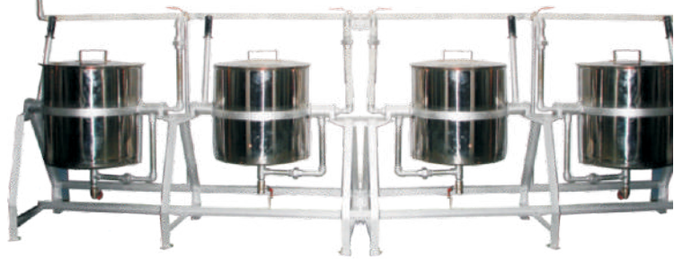
69 STEAM COOKING SYSTEM VESSELS
